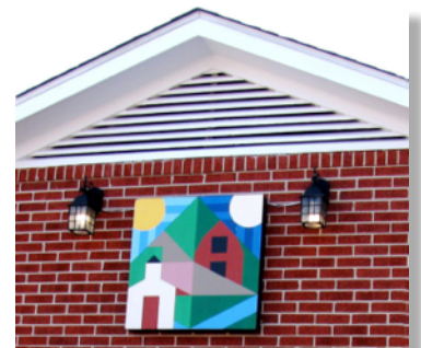
The eaves and upper arch frame of the Fellowship Hall are noticeably cleaner and whiter.
