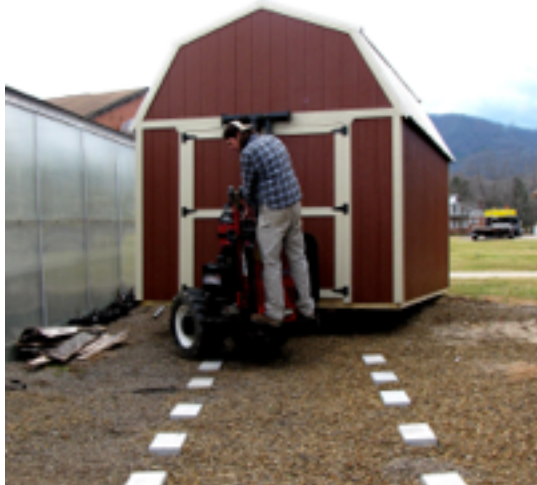
The storage unit is pulled into its final resting place next to the greenhouse.
