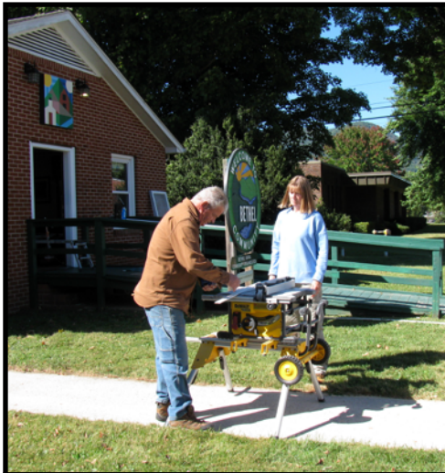
BRCO members Brent McKee and Gina Valeri brought their portable table saw and all of the necessary tools and materials.
